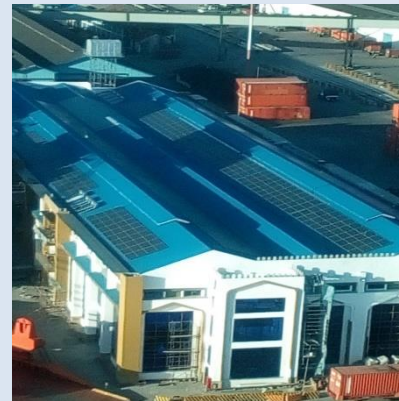
Roof-top solar PV installed at cruise ship terminal
