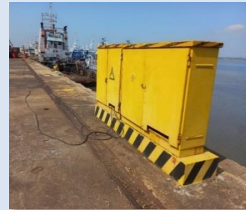
Source supplying electricity to boats when berthed
