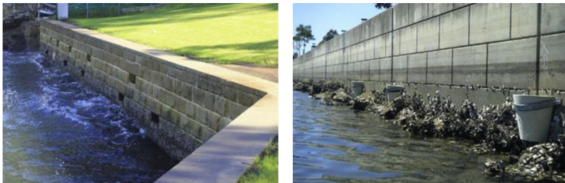
Figure C.7 Example of cavity pools (left) and flowerpots (right) on vertical seawalls (source: Morris et al. 2018)
