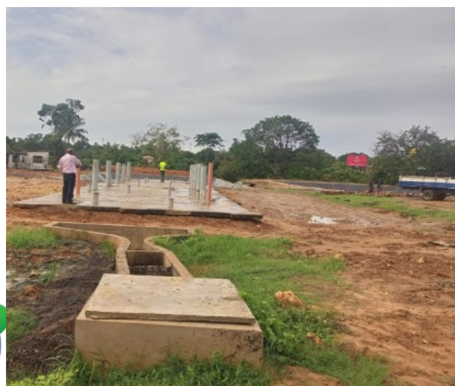
1. Anaerobic baffled reactor
