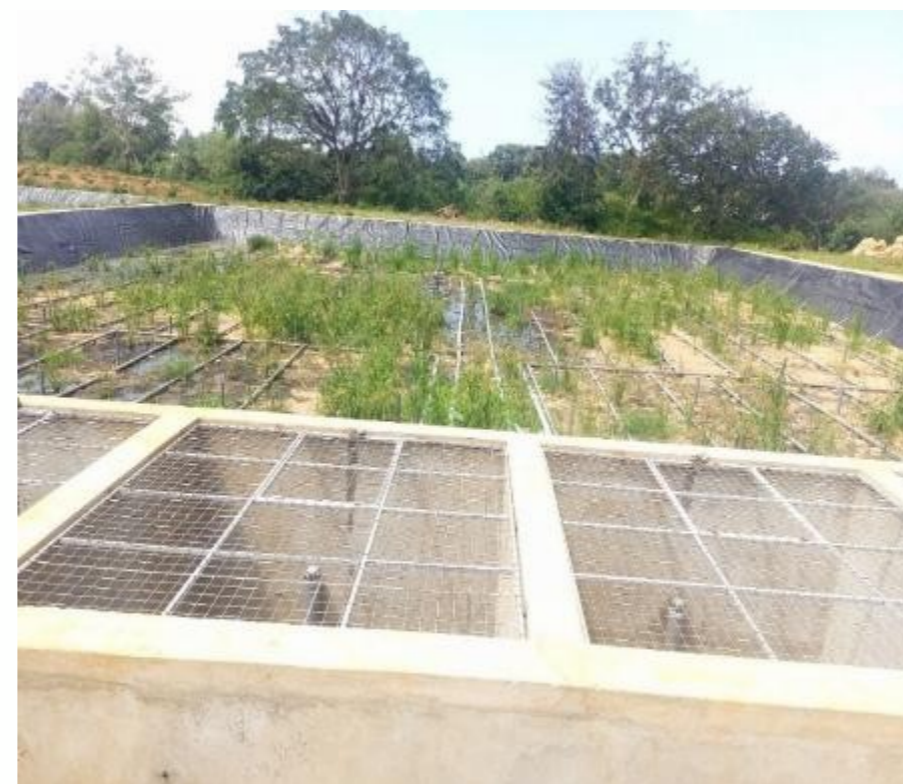
3. Vertical Flow Reed Bed (VFRB)
