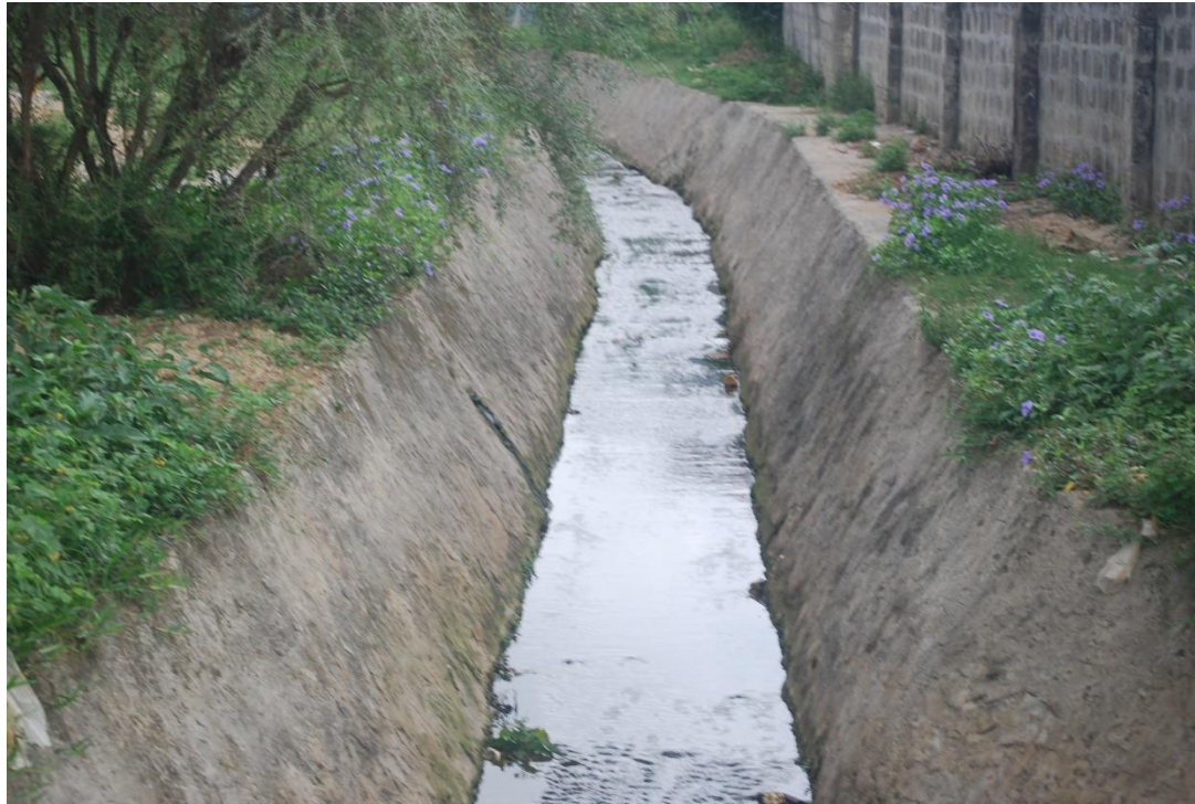
STORM WATER DRAIN TODAY
