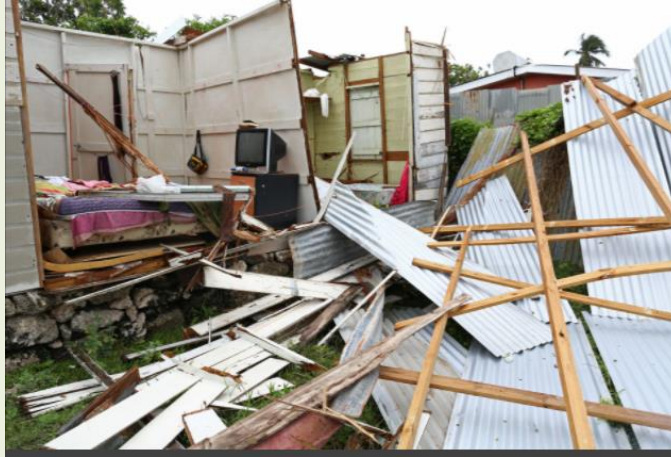
Damage caused to a house in Barbados (REUTERS/Nigel Browne)
