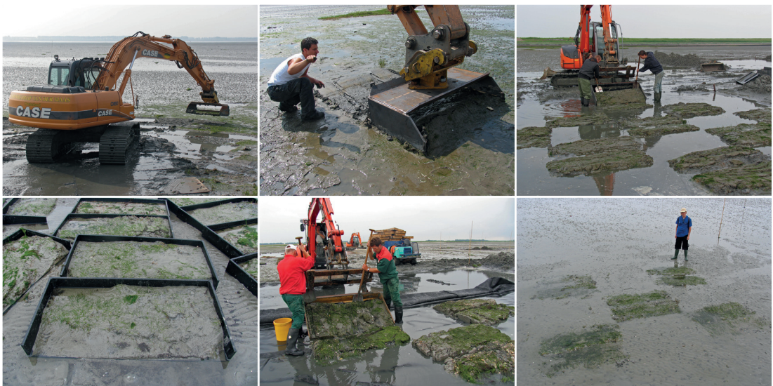
Plate 16. Photographic impression of the sod relocation method at the intertidal sites in the Eastern Scheldt, showing the modified backhoe scraping technique and transplant relocation.
